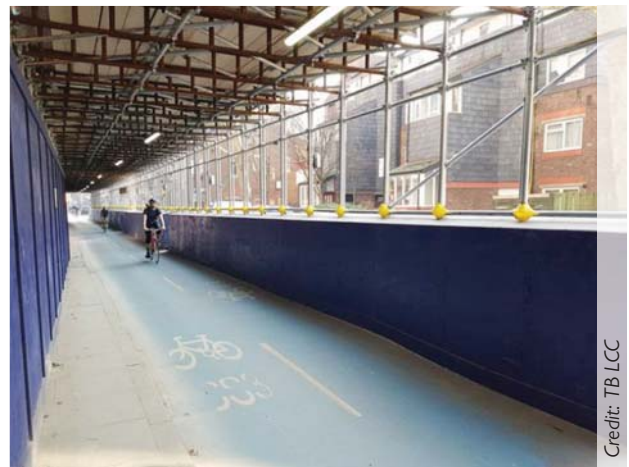
A cycle tunnel has been used here to avoid diversions and the need for cyclists to dismount
